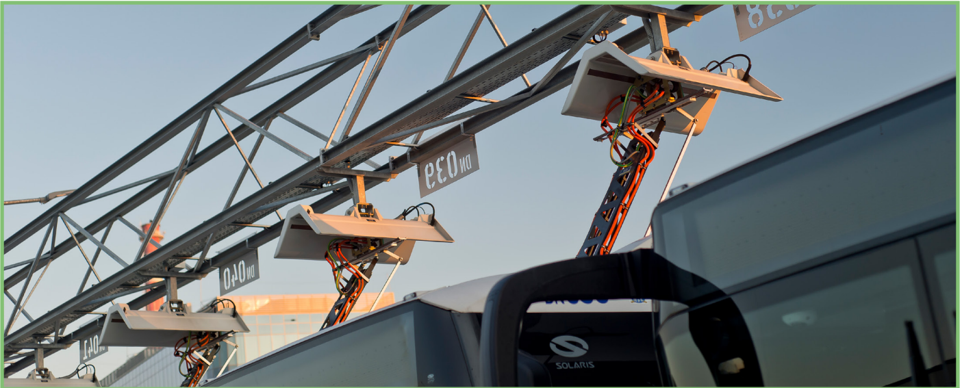
Electric buses equipped with roof-mounted pantographs stop under the charging station where the pantograph extends, connects to the charging station and charges the batteries
